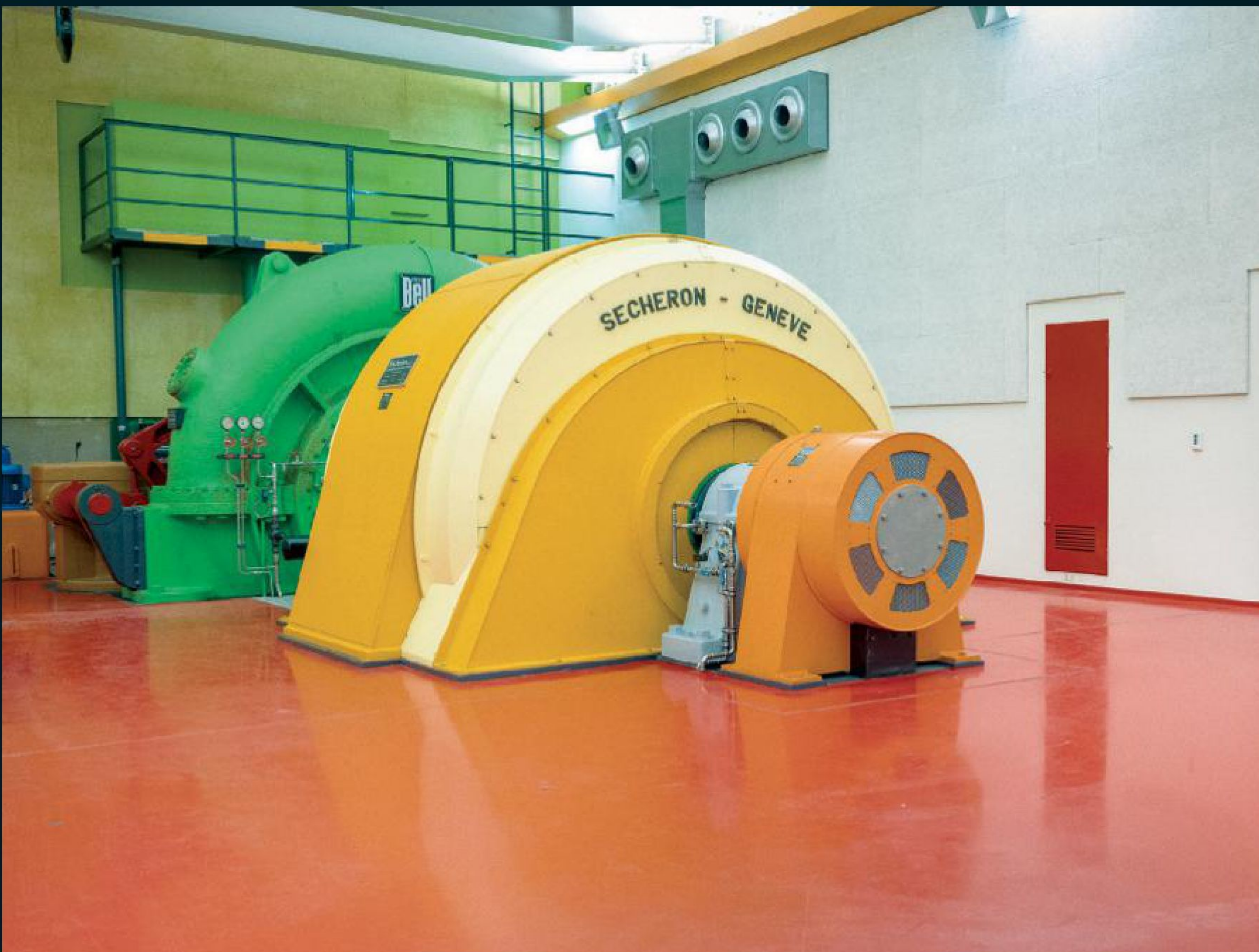
Located in the Italian-speaking canton of Ticino, the Luzzone dam is best known for its exterior. The world's highest artificial climbing wall rises 541 feet and features more than 650 man-made holds. Fewer see the interior of the dam, completed in 1963, and its pop art palette.
