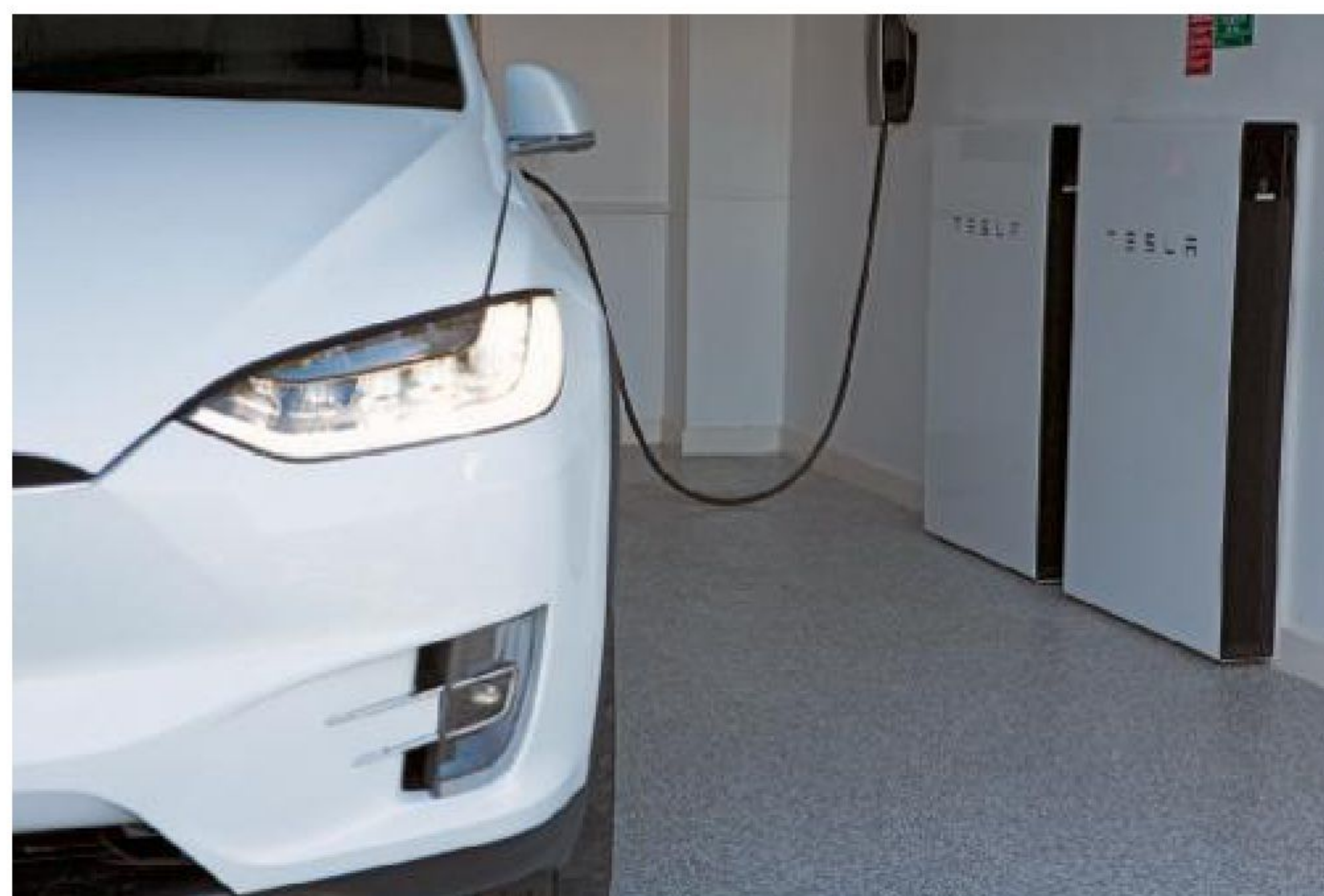
A Tesla Model X SUV fuels up at Amileka, a secluded holiday villa on Australia's eastern coast. On the building's roof, 33 solar panels collect the sun's energy, which is stored in Powerwall units and can be used to power the five-bedroom home and recharge electric vehicles.
